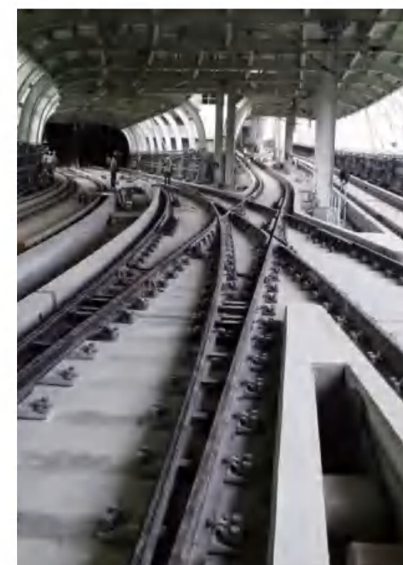
香港地铁道岔 Turnouts for Hong Kong metro
