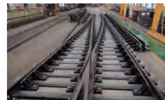
太原地铁新型减振道岔 Taiyuan Metro (New Type vibration reduction turnouts)
