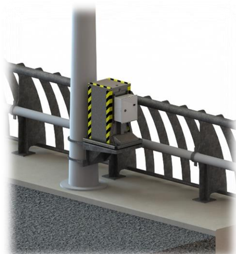
Main supply unit (inox) on power grid pillar (lifted from the ground)
